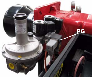
Fig. 29 - Gas pressure switch
