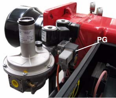
Fig. 22 - Gas pressure switch
